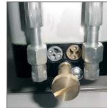
By-pass valves Válvulas by-pass
