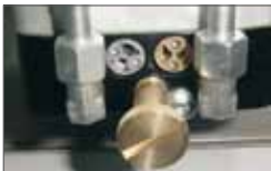
By pass valves
